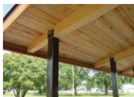
Steel Columns Powder coated steel columns
